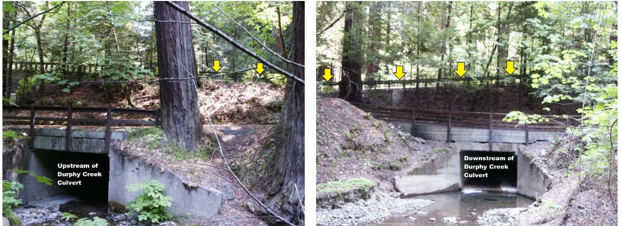
Figure 3.10 Durphy Creek Riparian Areas (yellow arrows show guardrail to be replaced with transition barriers and crash cushions)
