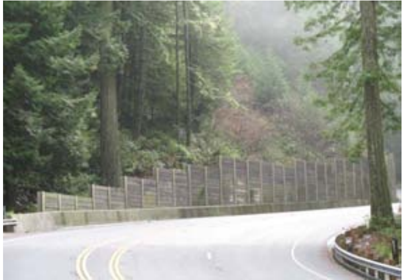
Similar type of retaining wall located in Del Norte Redwoods State Park
