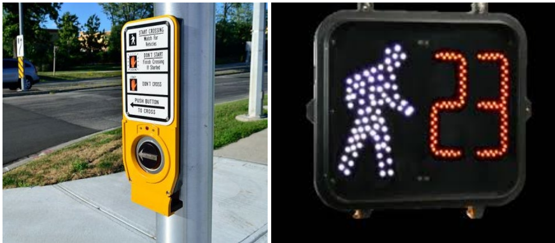
Figure 1.3.2-8: Accessible Pedestrian Signal System (left) and Countdown Pedestrian Signal System (right)
