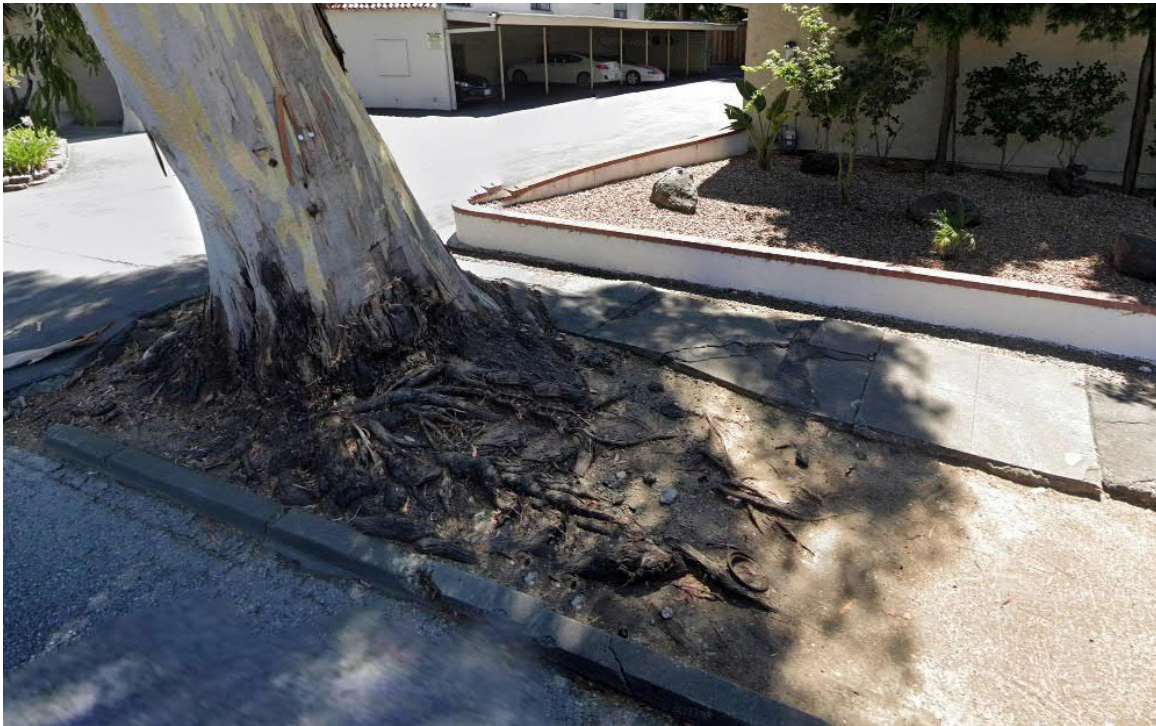
Figure 1.3.2-6: Narrow sidewalk between a tree and a retaining wall along El Camino Real between Carmelita Avenue and Sanchez Avenue
