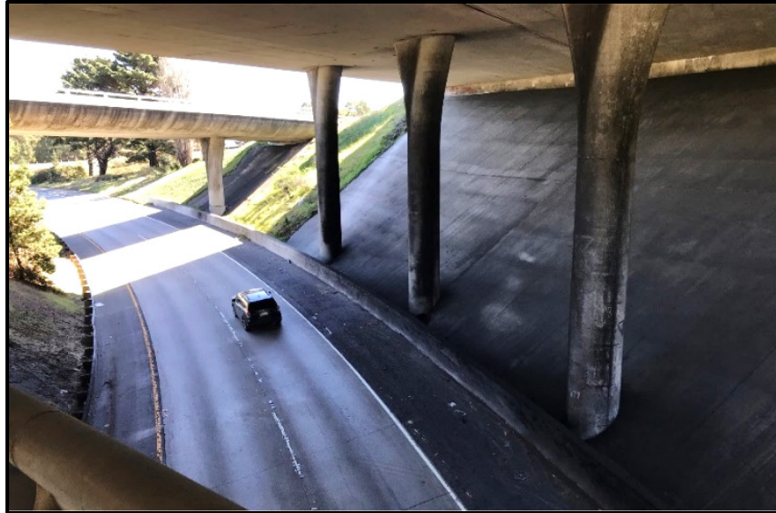
Photo 9: I-280/I-380 Separation Bridge; View of EB I-380 from a staging area under the I-280 Bridge
