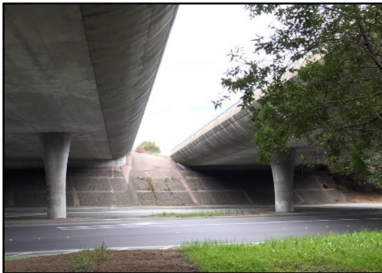
Photo 1: Alpine Road UC (L/R) Bridges; View north of Abutment 5, Bent 4, and Alpine Road
