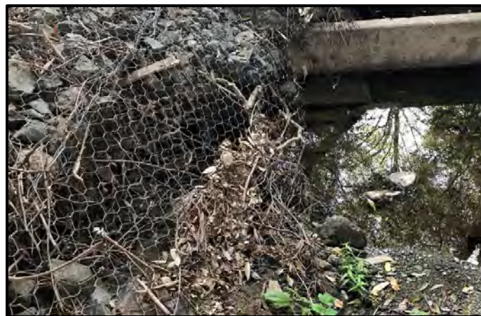
Photo 5: Alpine Road UC (L/R) Bridges; View south east of the gabion mattress (left side) and a weir (upper right side)
