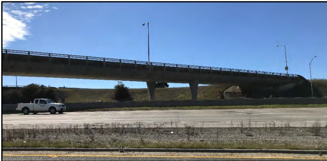
Photo 7: Sand Hill Road OC (South and North); View south east of Sand Hill Road OC North Bridge (Bent 2 and Abutment 1)
