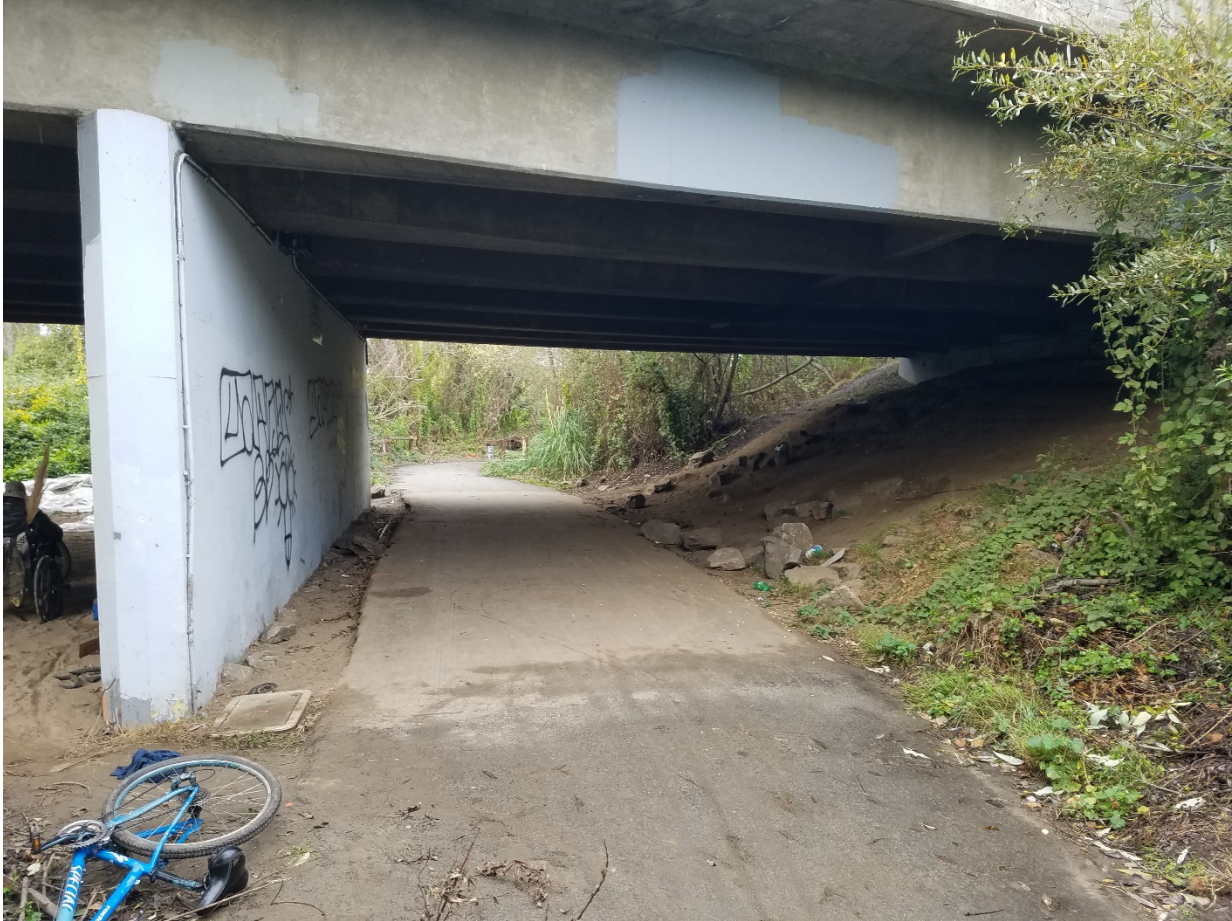
Figure 6 Portion of Naomi Partridge Trail below the Southbound Pilarcitos Creek Bridge between Pier 3 and Abutment 4
