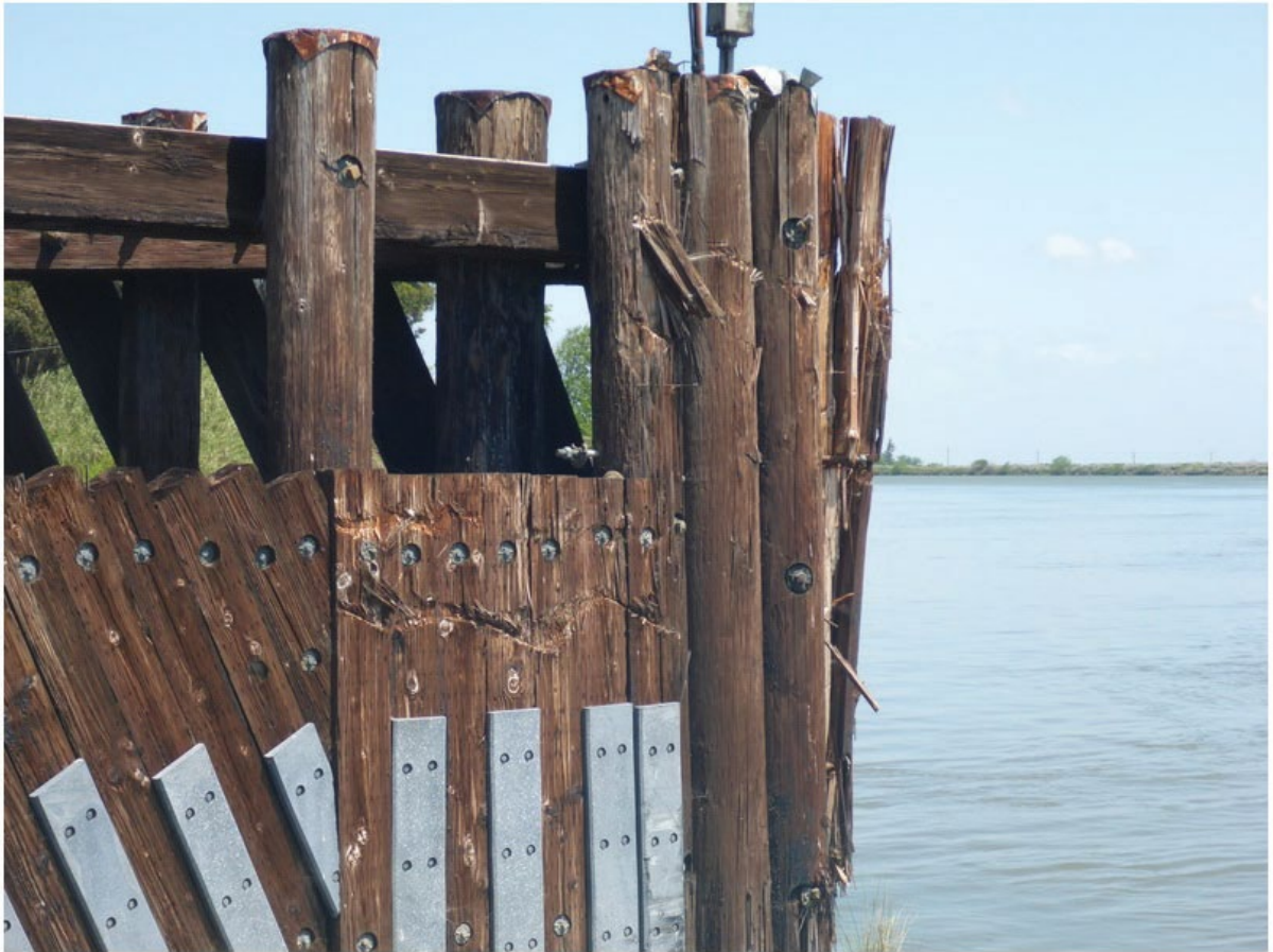
Figure 1-2. Damaged End Piles of the Fender System in Rio Vista
