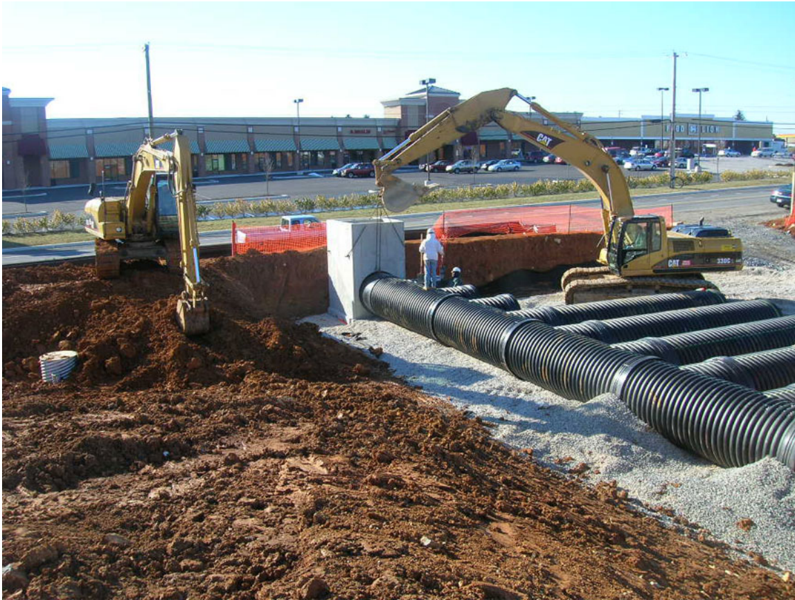
Figure 4-1. Example of Perforated HDPE Pipe installation, Photo from Plastic Pipe Institute website.
