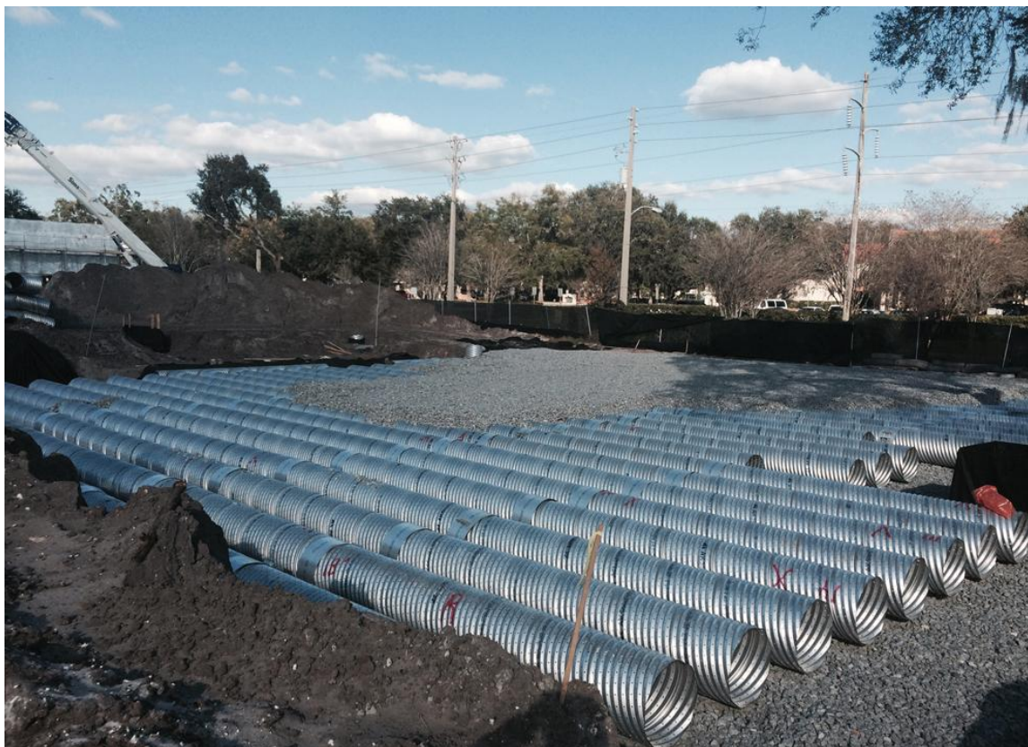
Figure 4-2. Example of Perforated Metal Pipe installation, Photo from Storm Water Solutions Magazine website.
