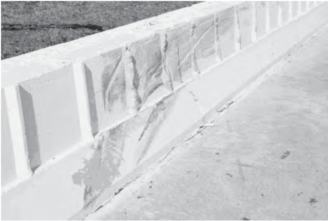
Figure 72. Barrier damage for Crash Test 3.
