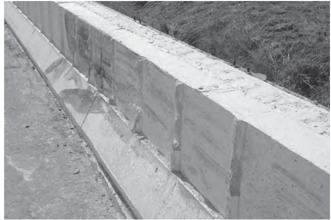
Figure 68. Barrier damage for Crash Test 1.
