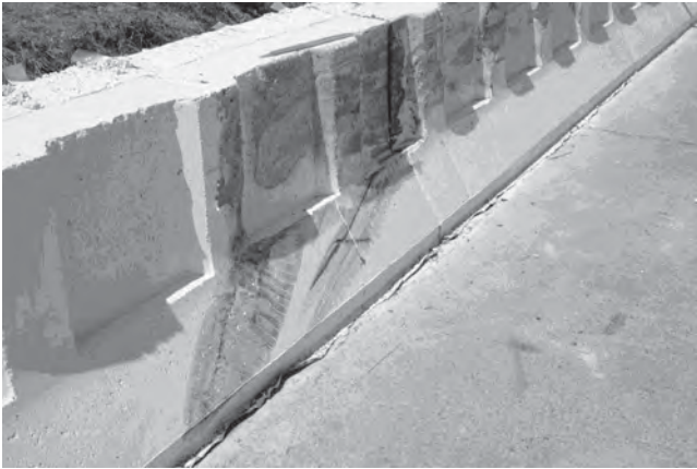
Figure 81. Barrier damage for Crash Test 7.
