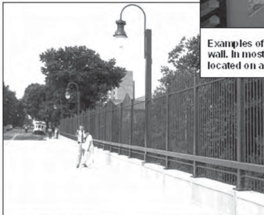
This rail is another example of a popular method to create attractive rails in urban areas. This Virginia project is located in low-traffic-speed street.
