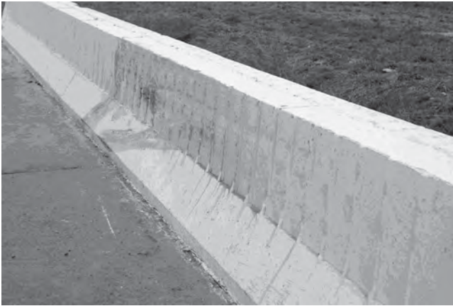
Figure 70. Barrier damage for Crash Test 2.
