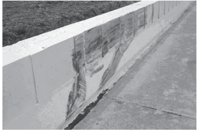
Figure 76. Barrier damage for Crash Test 5.
