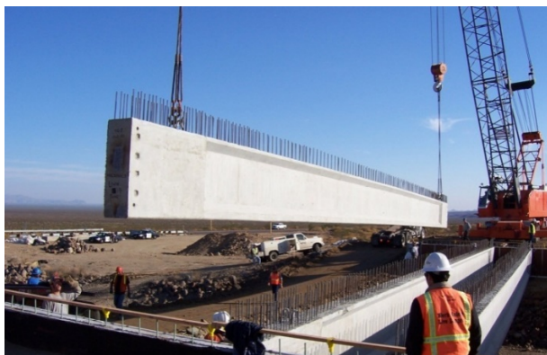
Figure 5.3.3-1 Single-Span I Beam Lowered onto Abutments at Mustang Wash Bridge (Bridge No. 54-1279L, Caltrans)
