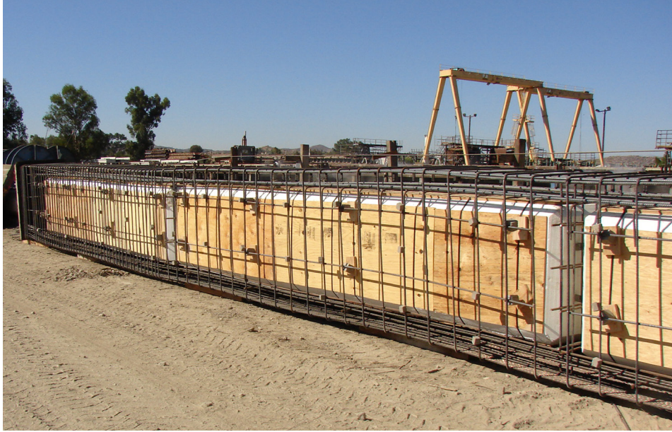
Figure 5.4-2 Precast Box Girder Void Forms, Strand, and Reinforcing Steel (Courtesy of TYLin)
