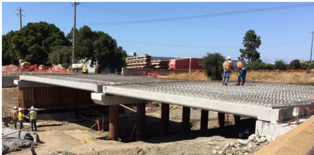
Figure 5.5-4 Voided Slabs with Stirrups Extending into a Cast-in-Place Concrete Deck (Courtesy of Kie-Con)
