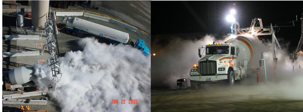
Figure 7-13. Liquid Nitrogen Coolant Injection.
