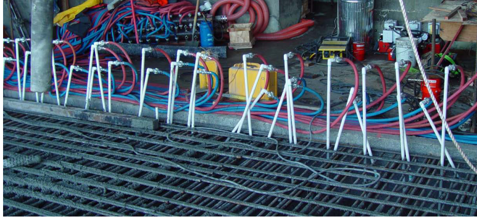
Figure 7-26. Soffit Cooling Pipe Manifold.
