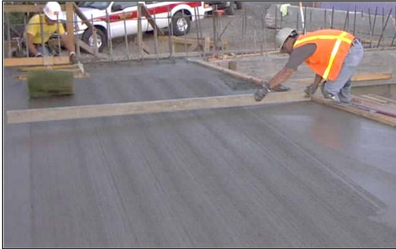
Figure 2.2-2. Finisher Checking the Freshly Placed Deck Concrete Near the Expansion Joint Blockout.
