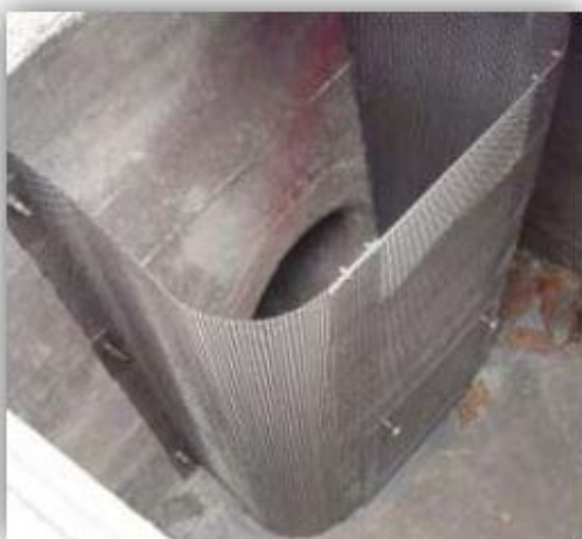
Catch Basin Outlet Screen
