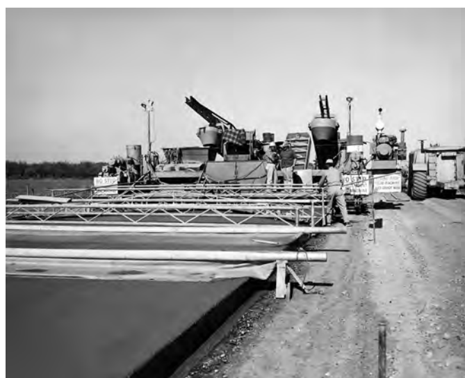
Figure 140. Slip-form concrete base being laid near Winters, California, along SR 205 (Caltrans Transportation Library, Sacramento).
