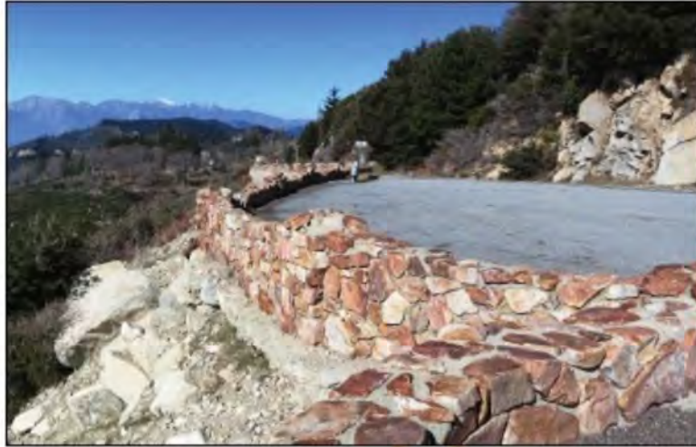
Rubble masonry parapet walls at Strawberry Scenic Overlook, constructed of Saragossa quartzite. View to the west at P.M. 21.5.
