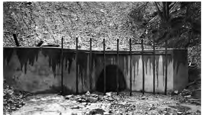
Figure 111. Concrete headwall on a highway culvert in Mendocino County, 1950 (Caltrans Transportation Library, Sacramento).
