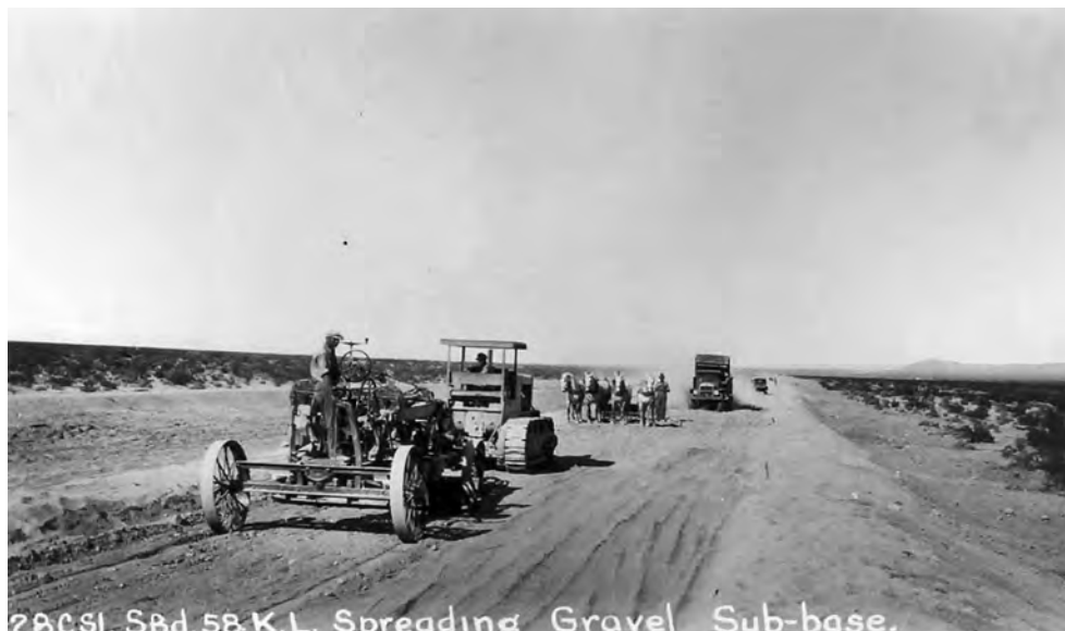
Figure 139. Construction of San Bernardino SR 40, 1931 (Contract No. 28CS1). Note the use of both animals and mechanical equipment in the grading and preparation of the road surface (Caltrans Transportation Library, Sacramento).
