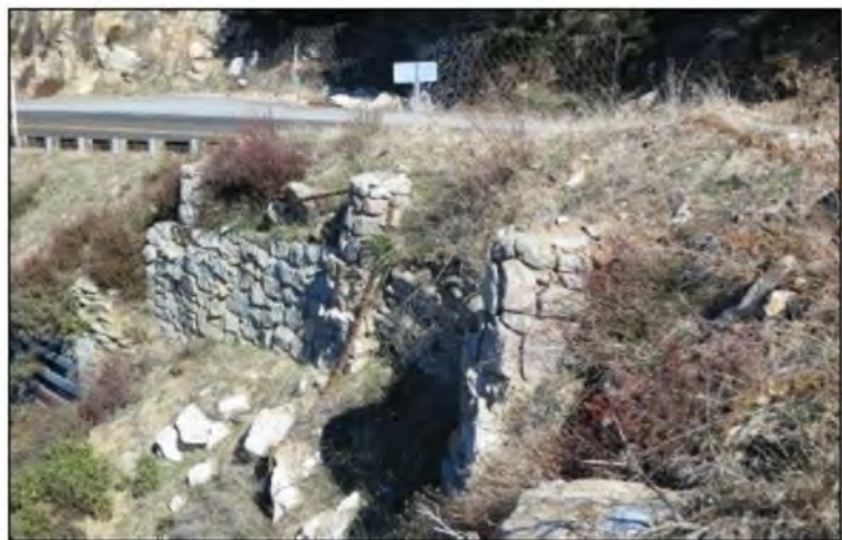
Inundated rubble masonry "pier-and-chain" guardrails atop rock retaining wall, inundated by slide fill. View west at P.M. 18.85.
