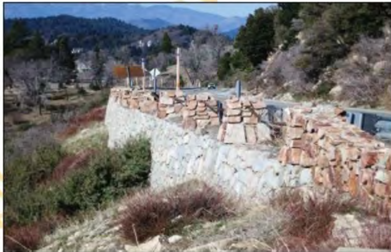
Rubble masonry "pier-and-chain" guardrails atop rock retaining wall, view west at P.M. 21.
