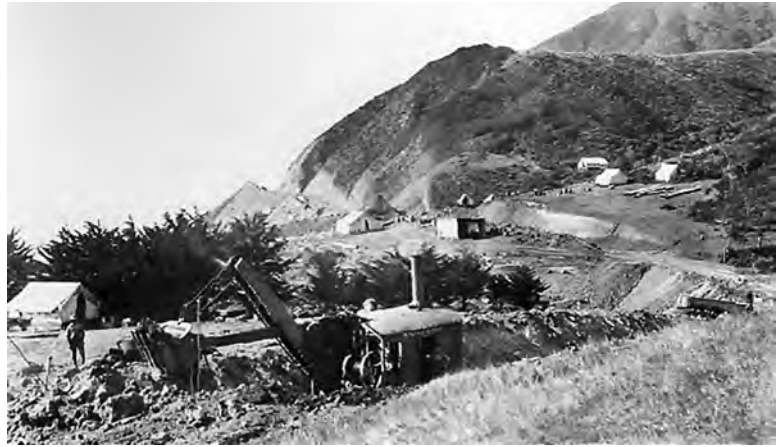
Figure 129. Rural highway in San Luis Obispo County under construction, 1923 (California Division of Highways, San Luis Obispo County (SLO) 56A, Contract 331).
