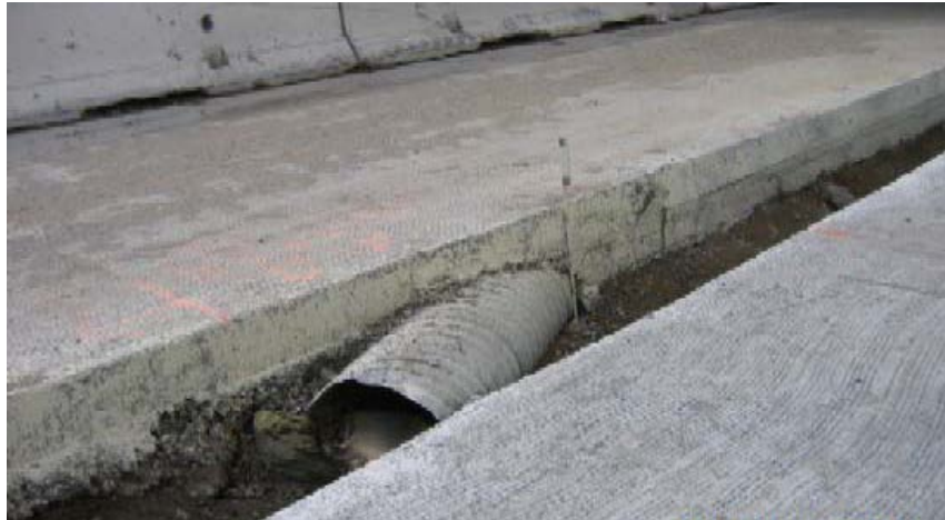
Figure 210–7: Concrete pavement structure with inadequate cover
