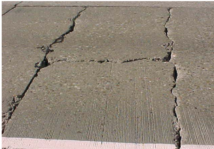
Figure 320-4: Replace slab – 3 rd stage cracking \geq \frac{3}{4} " wide with minor spalling
