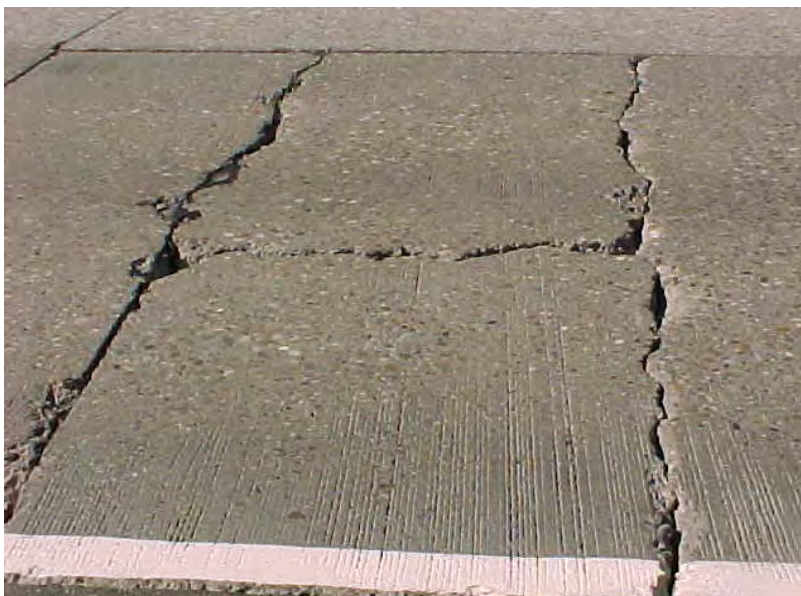
Figure 410-3: 3 rd stage JPCP cracking
