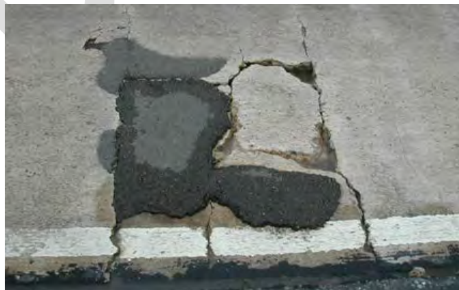
Figure 380-1: Typical CRCP punchout distress (FHWA)
