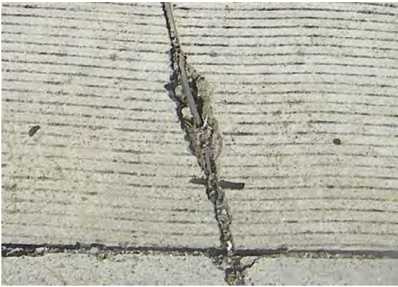
a) Seals not maintained or replaced
