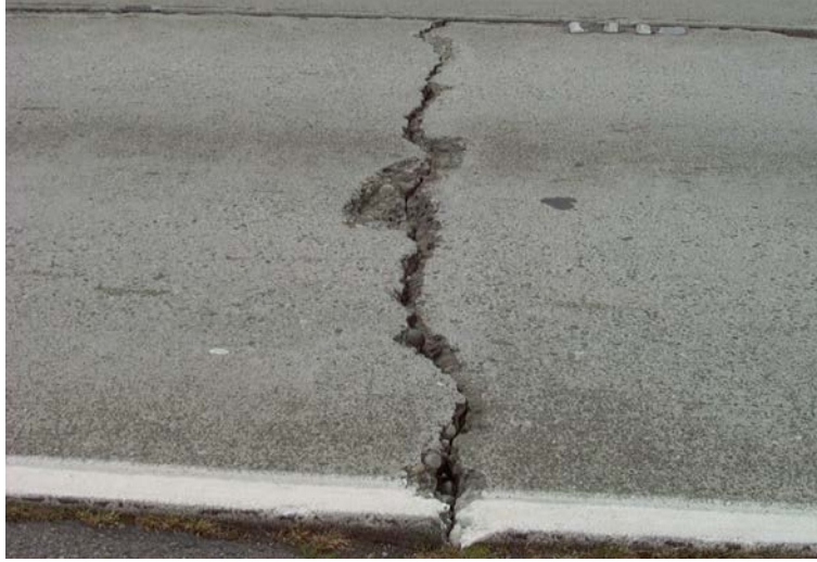
Figure 320-3: Replace slab – transverse crack \geq \frac{3}{4} " wide with spalling
