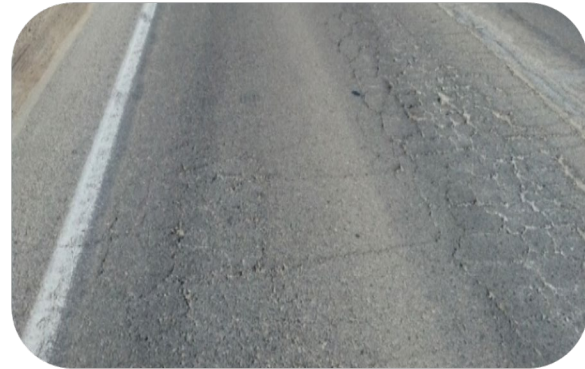
Alligator B Cracking
