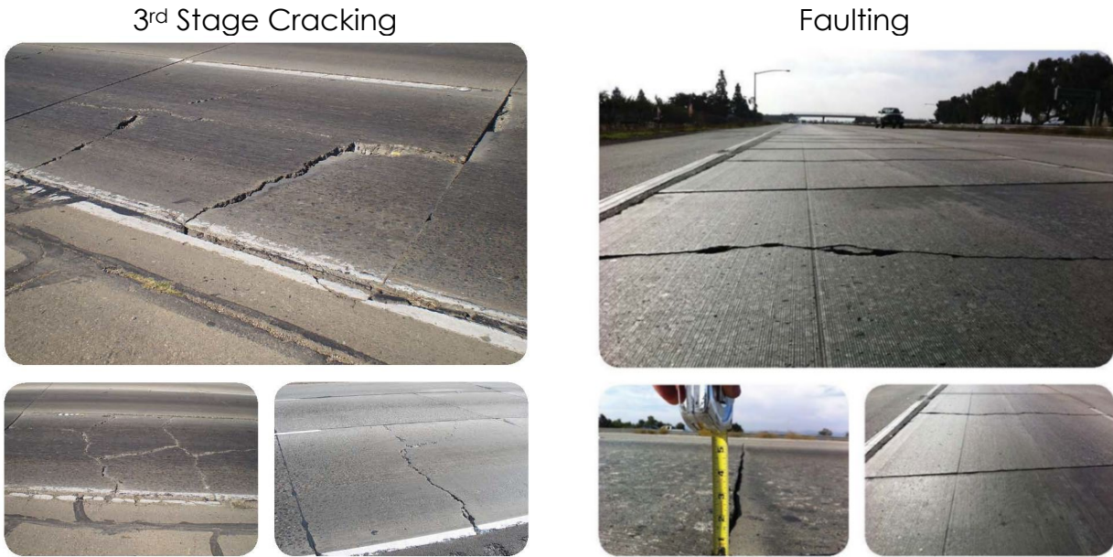
FIGURE 4. EXAMPLES OF DISTRESS FOR CONCRETE PAVEMENT
