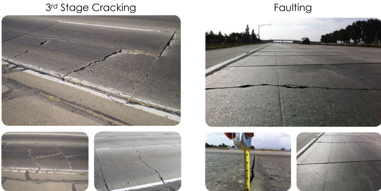
FIGURE 4. EXAMPLES OF DISTRESS FOR CONCRETE PAVEMENT
