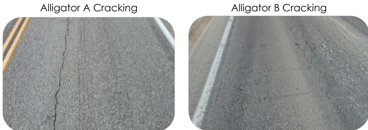
FIGURE 3. EXAMPLES OF DISTRESS FOR ASPHALT PAVEMENT
