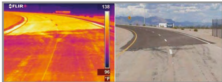
Thermal infrared (left) and visible (right) images of a road with light and dark segments. The infrared image shows that the light segment (bottom) is about 17°C (30°F) cooler than the dark segment (top). (Image courtesy of Larry Scofield, APCA)
