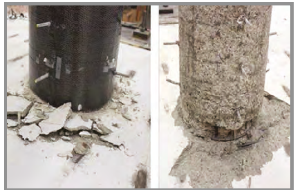
Cap beam concrete crushing and column flexural cracks (CFRP jacket removed) after hybrid simulation tests
