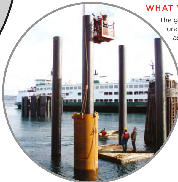
Surrounding a 30-inch-diameter pile with a temporary double-walled steel tube to suppress noise
