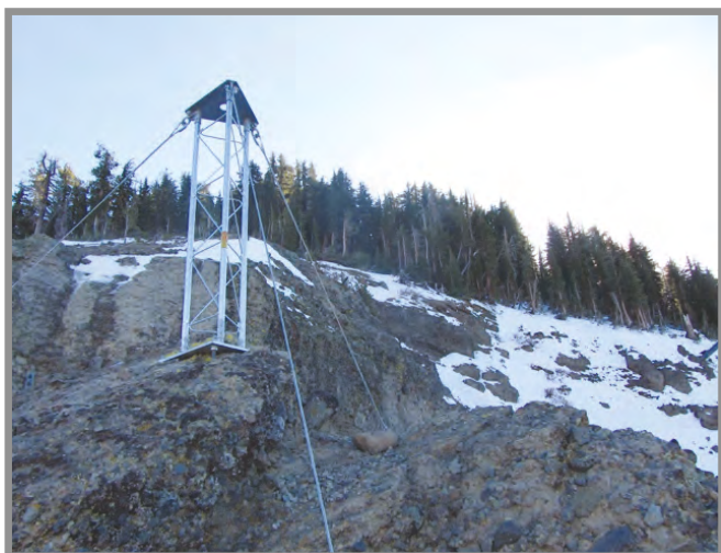
Tower installed on Carson Spur to hold the instrumentation equipment
