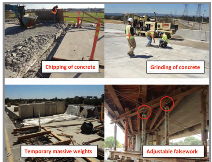
Hinge curl remedial measures
