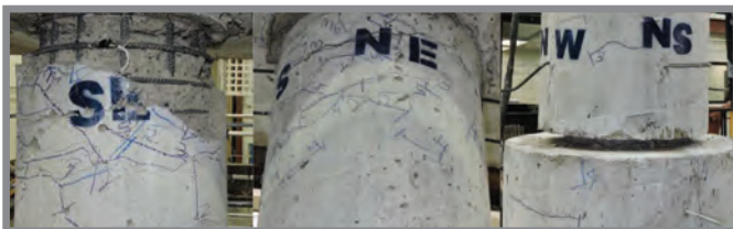
Damage after the final test: (left) cast-in-place column; (center) precast column with ECC; (right) precast column with rebar
