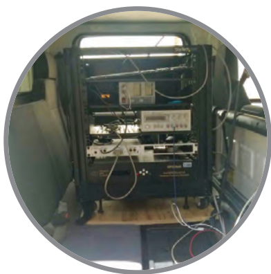
Server racks holding the equipment
