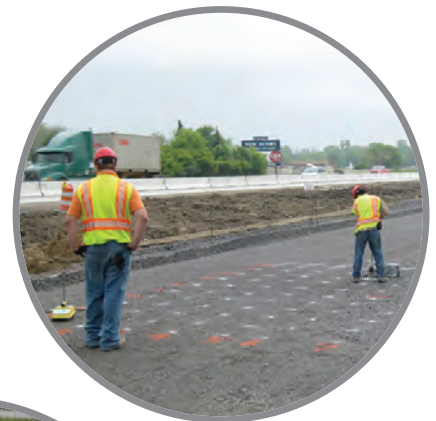
Field testing on a dense grid to capture the spatial variability of foundation layer support conditions
