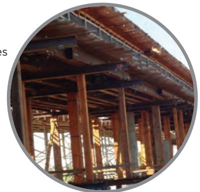
Left: Constructing the temporary structure used to support the span (falsework) for the Del Paso Park overhead in Sacramento
