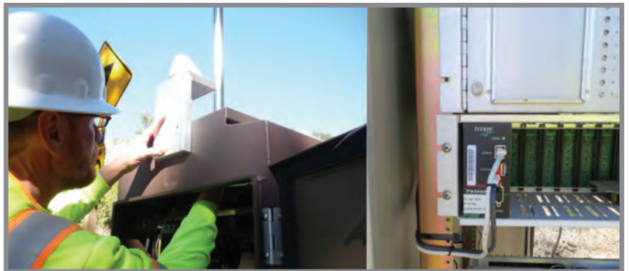
The Bluetooth reader system consists of the Iteris Bluetooth detector unit, a radio transmission device, RF cable, and antenna.
