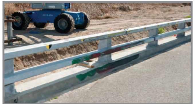
Damage to the barrier
