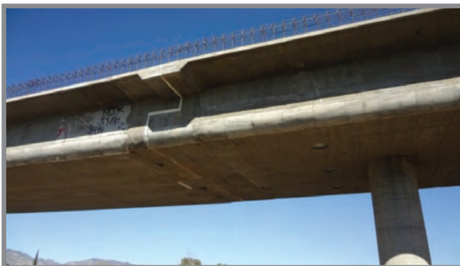
In-span hinge of a cast-in-place, prestressed box girder bridge on the N170-N5 connector in Los Angeles
