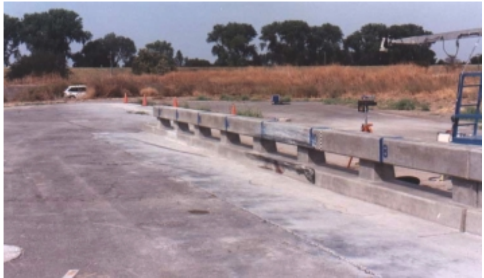
Figure 2-19 Post Impact View of Barrier and Vehicle 544
