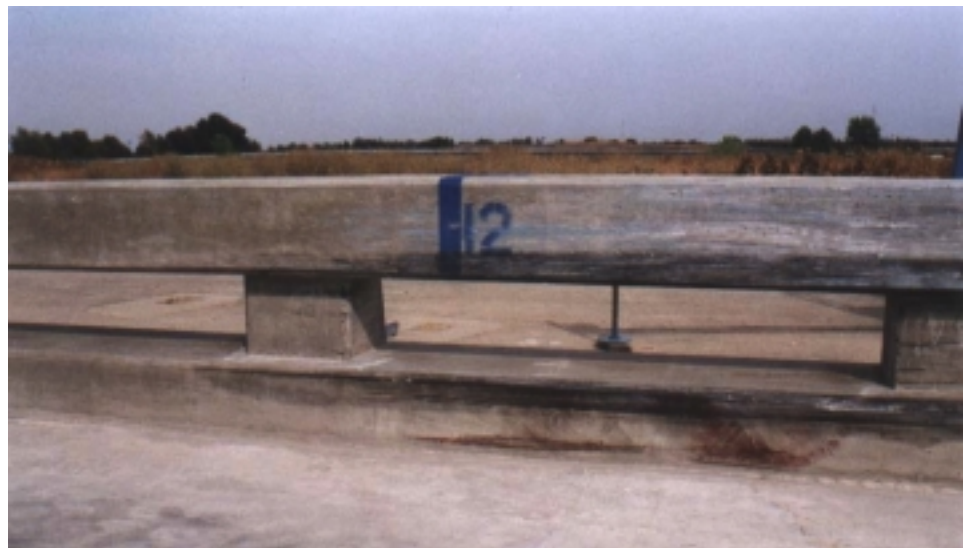
Figure 2-21 Post Impact Bridge Rail Scuff Marks Test 544
