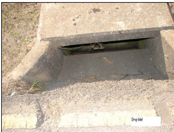
Functional Drop Inlet Condition - Do Not Count as Deficient
