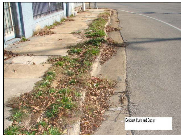
Deficient Curb and Gutter Condition - Count Linear Feet of Deficiency
