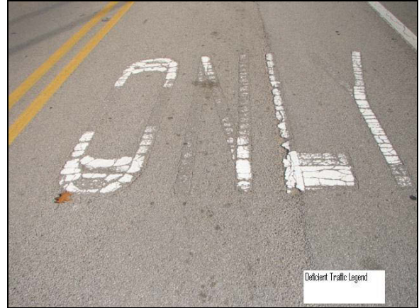
Deficient Pavement Legend Sample – Count as Deficient
