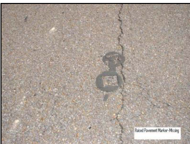
Missing Raised Pavement Marker – Count as Deficient
