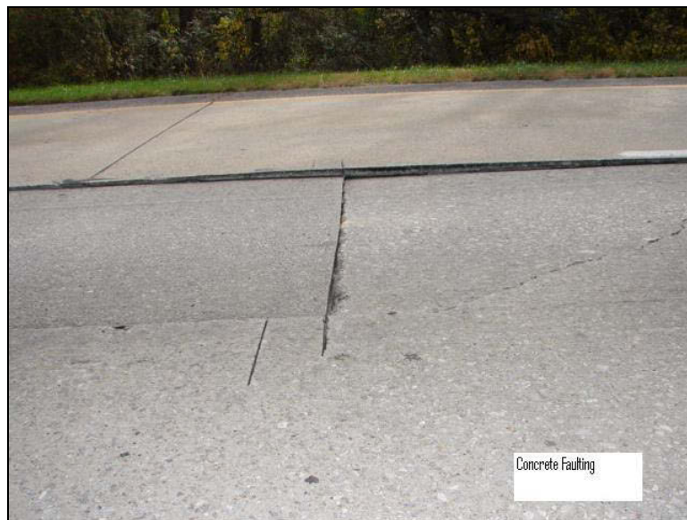
Sample Concrete Faulting
