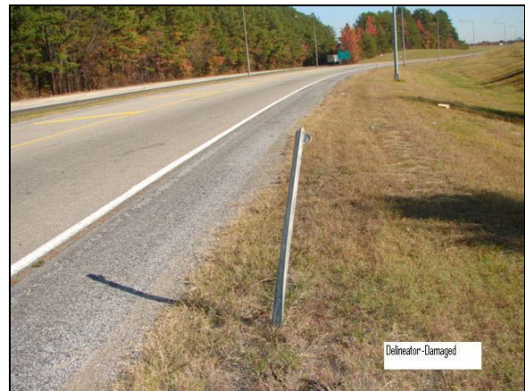
Deficient Delineator – Count as Deficient
