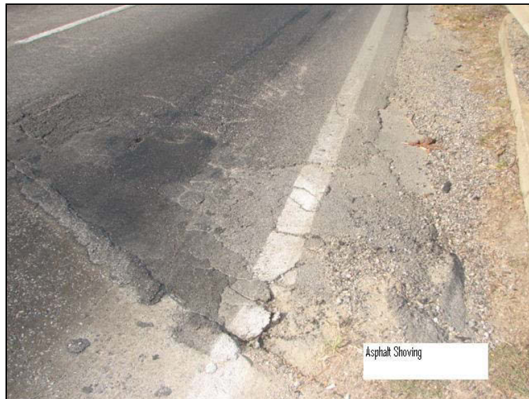
Sample Asphalt Shoving
