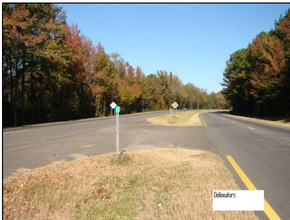
Functional Delineator – Do Not Count as Deficient
