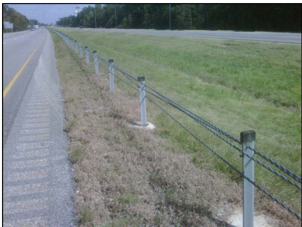
Functional Cable Rail Sample – Do Not Count as Deficient
