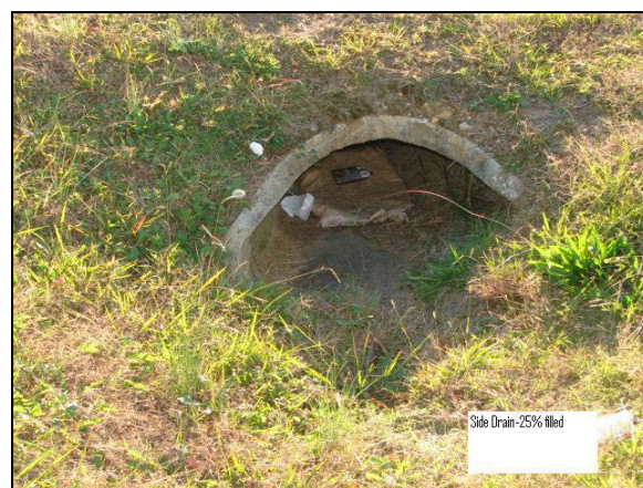
Deficient Side Drain Condition - Count as Deficient
