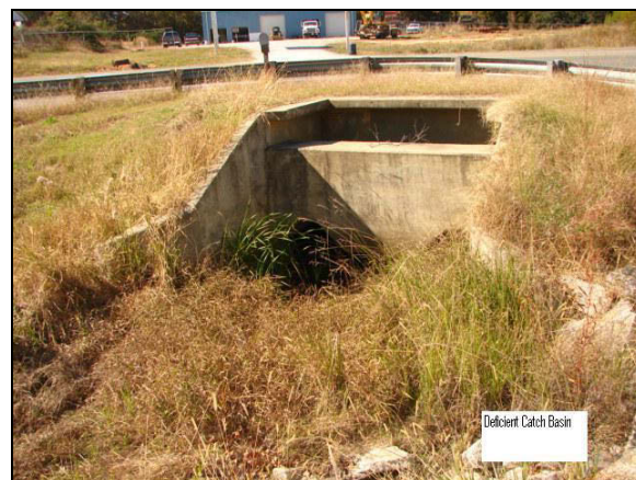
Deficient Catch Basin Condition - Count as Deficient
