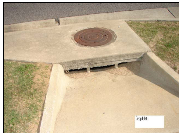
Deficient Drop Inlet Condition - Count as Deficient
