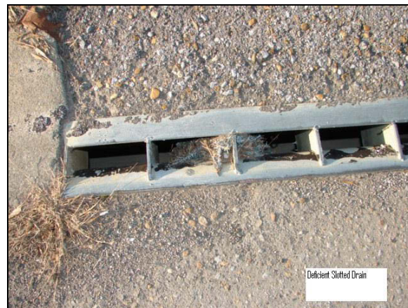
Deficient Slotted Drain Condition - Count as Deficient
