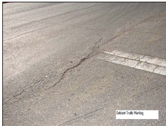
Deficient Pavement Marking Sample – Count as Deficient
