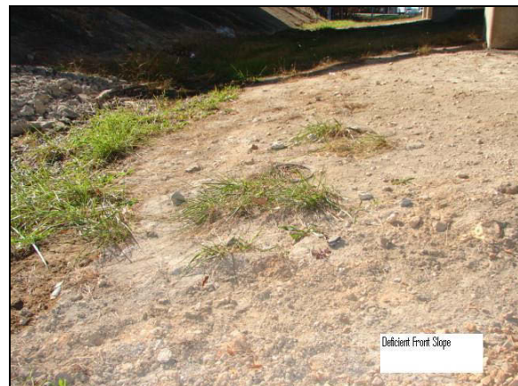
Deficient Front Slope Condition - Count Linear Feet of Deficiency
