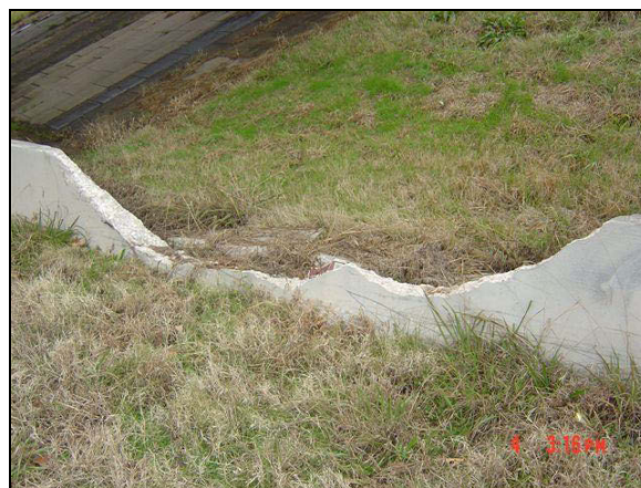
Deficient Barrier Wall Sample – Count Linear Feet of Deficiency
