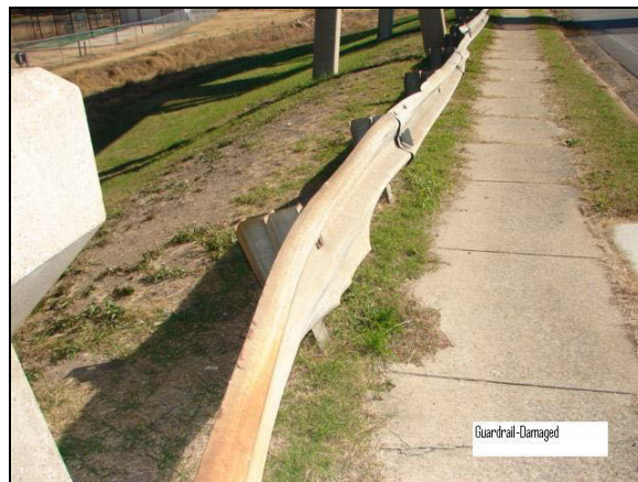
Deficient Guardrail Sample – Count Linear Feet of Deficiency
