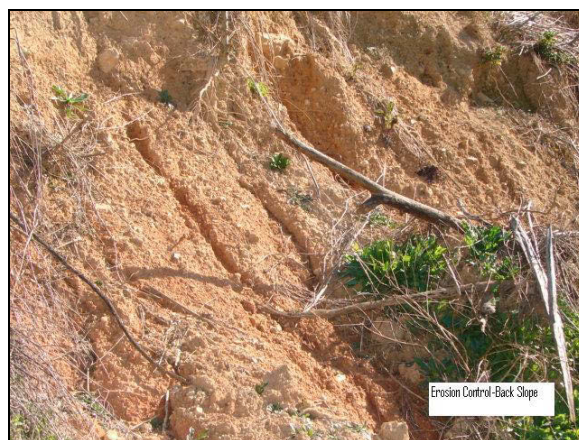
Deficient Back Slope Condition - Count Linear Feet of Deficiency
