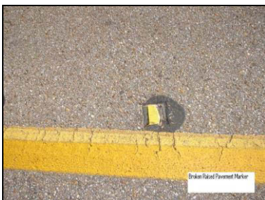
Damaged Raised Pavement Marker – Count as Deficient
