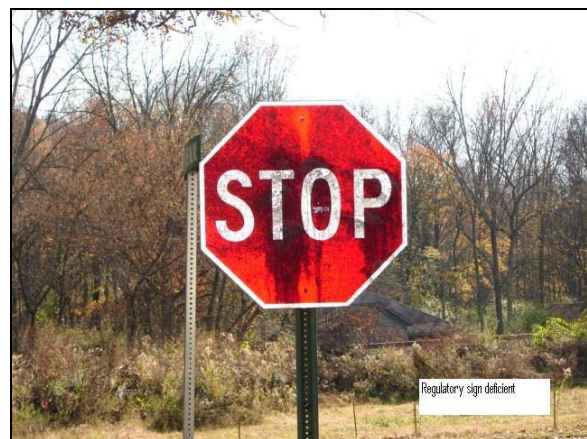
Deficient “Regulatory Sign” Sample – Count as Deficient
