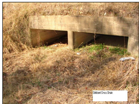
Deficient Cross Drain Condition - Count as Deficient
