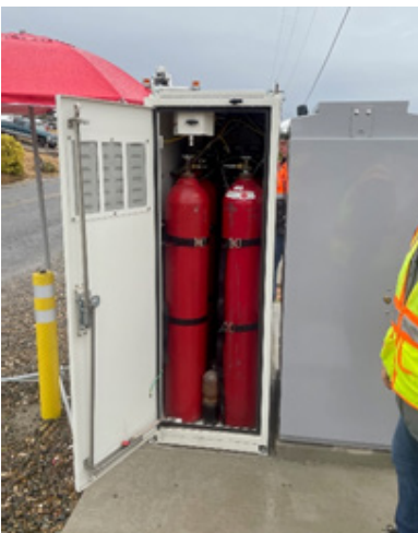
Image 2: Hydrogen Fuel Cylinder cabinet - Source: Caltrans
