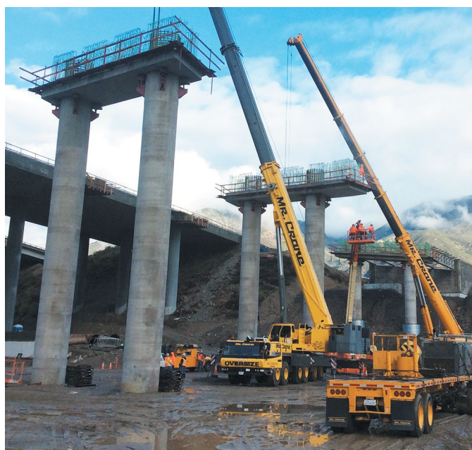
Precast bent cap beams are laid atop of bridge columns for what would be northbound I-15 to the southbound I-215 connector bridge.
