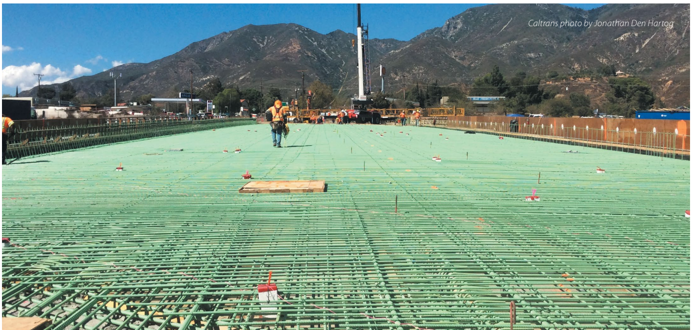
A series of reinforcing steel bars for the new Devore Road overcrossing bridge deck give off an almost water-like shimmer in the afternoon sun. The Cajon Pass and Devore Interchange projects took about three years to complete, and were completed on time and within budget.
