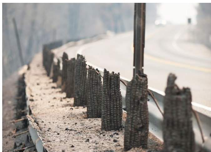
The Carr Fire on SR 299 burned right up to the road's edge, and in some spots jumped it, destroying guardrail, signs and pavement.
