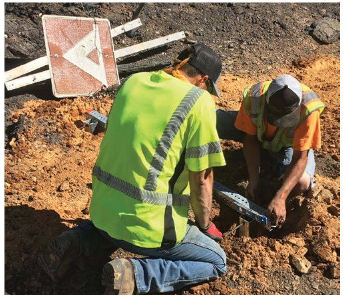
A contracting crew, under orders from Caltrans District 2, acted quickly to replace damaged signs along SR 299, near Whiskeytown.
