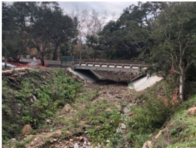
DAMAGE TORO CANYON CREEK BRIDGE SR 192 IN SANTA BARBARA COUNTY
