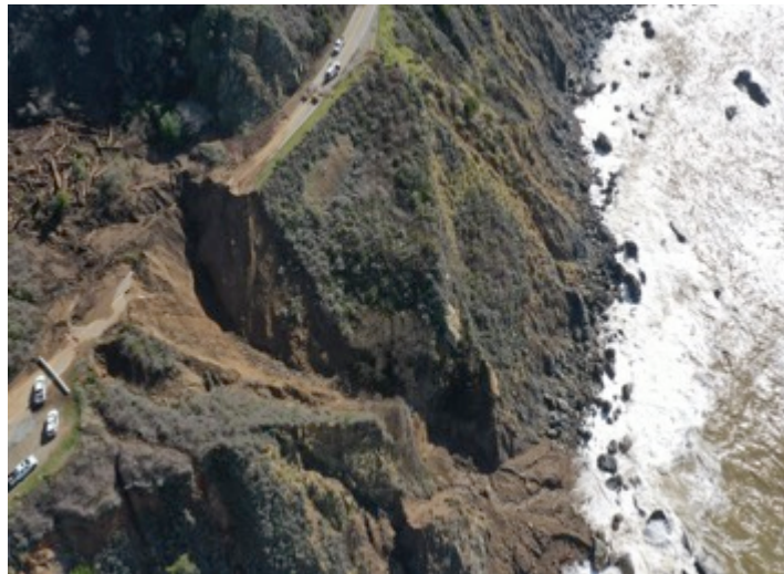
RAT CREEK MUDSLIDE DEBRIS FLOW SR 1 IN MONTEREY COUNTY
