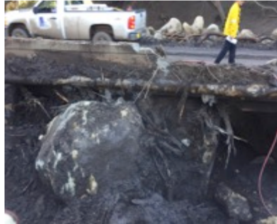
DAMAGE TO TORO CREEK BRIDGE CAUSES DETOURS SR 192 IN SANTA BARBARA COUNTY
