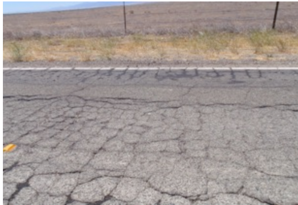
EXTREME HEAT CAUSES PAVEMENT DAMAGE, SR 58 IN SAN LUIS OBISPO COUNTY
