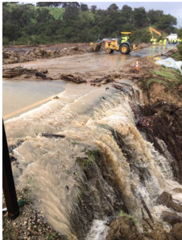
FLOODING DUE TO DEBRIS CLOGGED CULVERT SR 154 IN SANTA BARBARA COUNTY
