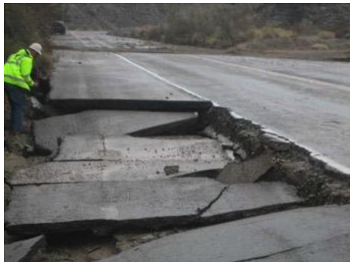
US-95 STORM EVENT AND CRACKED PAVEMENT
