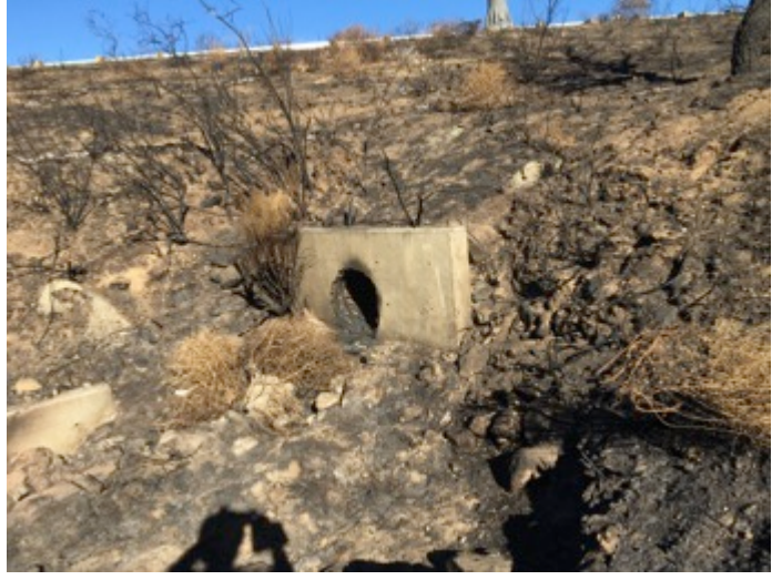
CULVERT AFTER A FIRE AT SR-91
