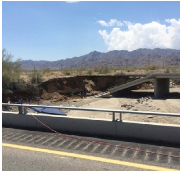
I-10 STORM DAMAGED BRIDGE
