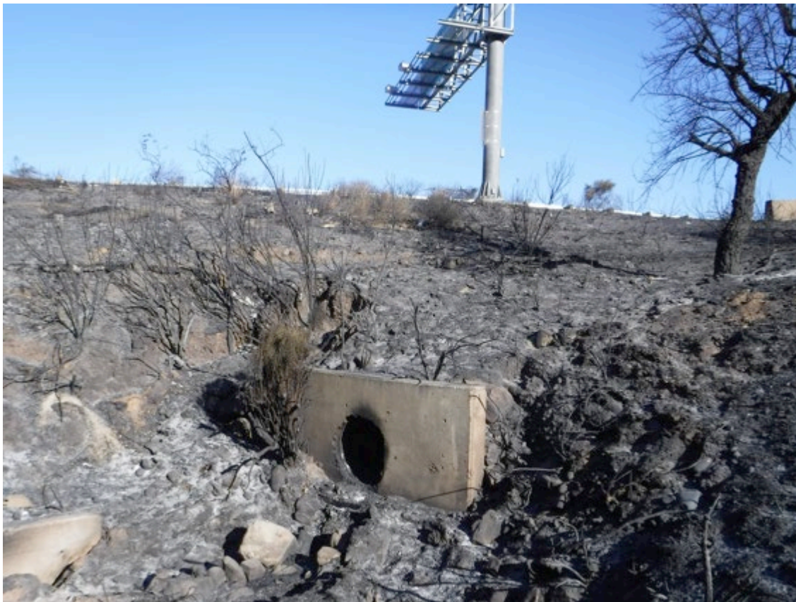
SR-91 CULVERT AFTER FIRE
